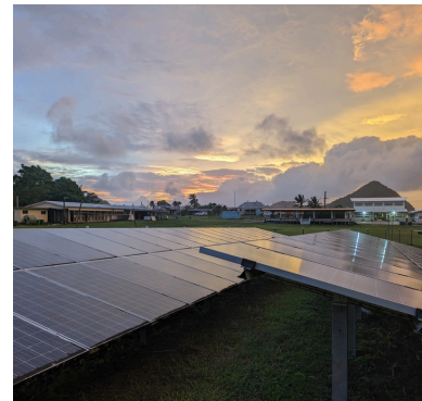
Rural Electrification Unit
